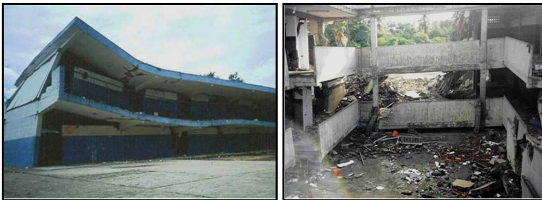
Figure 2. School buildings that collapsed during 07/09/1997 Cariaco Earthquake ( M_w=6.9 ): Valentin Valiente School (left) and Raimundo Martinez High School (right)
