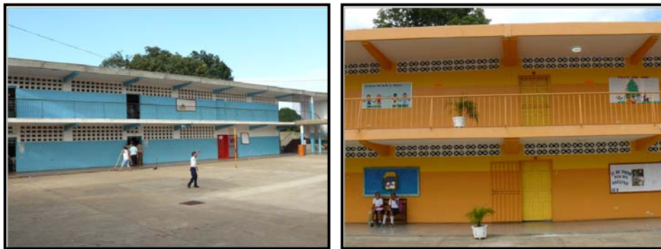
Figure 7. Old-Type I school buildings inspected in Sucre State
